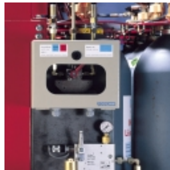
Switch over unit between main and reserve batteries
