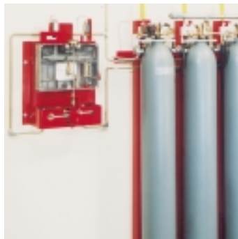
CO 2 storage battery with alarm control cylinder and mecha- nical delay device
